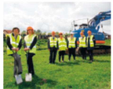
Two local residents who were affected by the flood cut the first turfs for the new scheme
